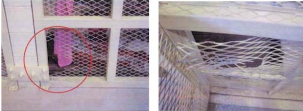
Detainees at Afghanistan's largest U.S.-built prison were able to literally kick through their poorly constructed cells, according to a new Pentagon report. Photo: Defense Department Inspector General
