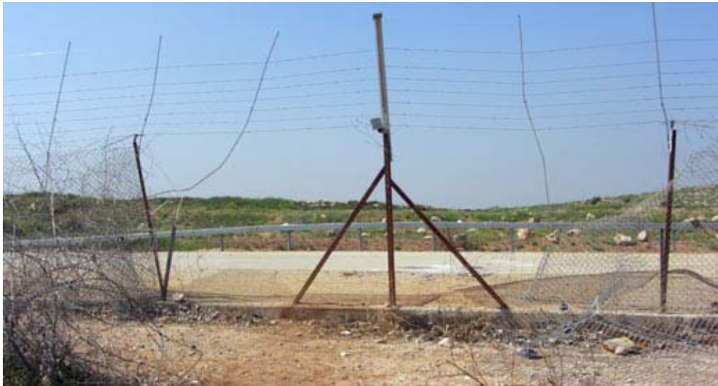
Breach in barrier where yusef was shot: Itamar Barak, B'Tselem, 20 March 2014
