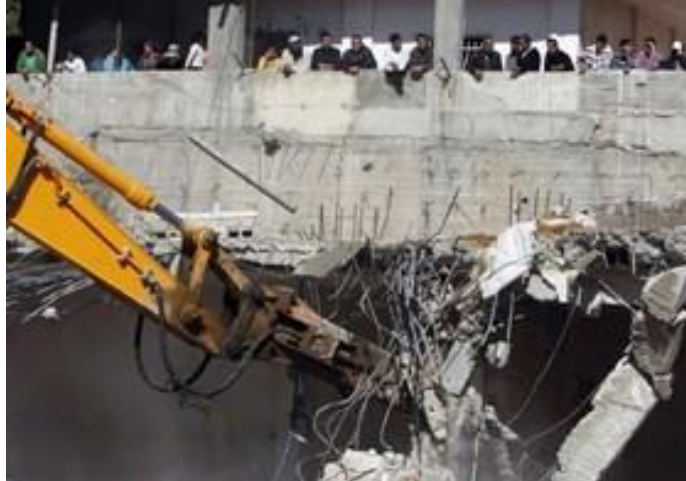
Israeli Occupation Forces (IOF) demolishes a Palestinian-owned factory and steel structure in Barta and Zebda towns southeast of Jenin. (Photo: PIC)
