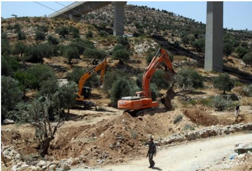
An Israeli excavator uproots olive trees to make way for Israel's controversial separation barrier, in the West Bank town of Beit Jala on August 17, 2015. (AFP/File Musa al-Shaer)
