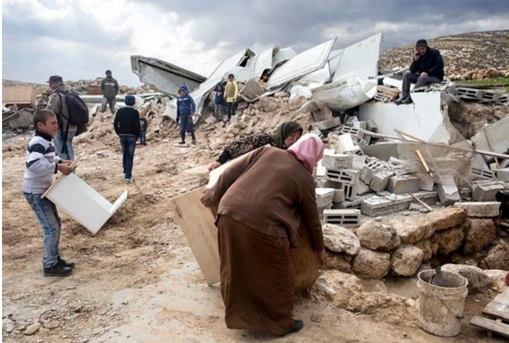
Villagers in Khirbet Jenbah rescue furniture following house demolitions. More than 80 villagers lost their homes in a single morning. Photograph: Peter Beaumont for the Guardian
