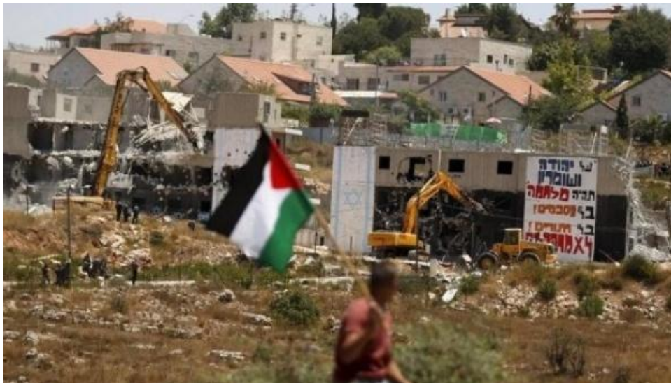
A Palestinian flag flies as Israeli heavy machinery demolish Palestinian apartment blocs at the West Bank Jewish settlement of Beit El July 29, 2015. Photo: Reuters
