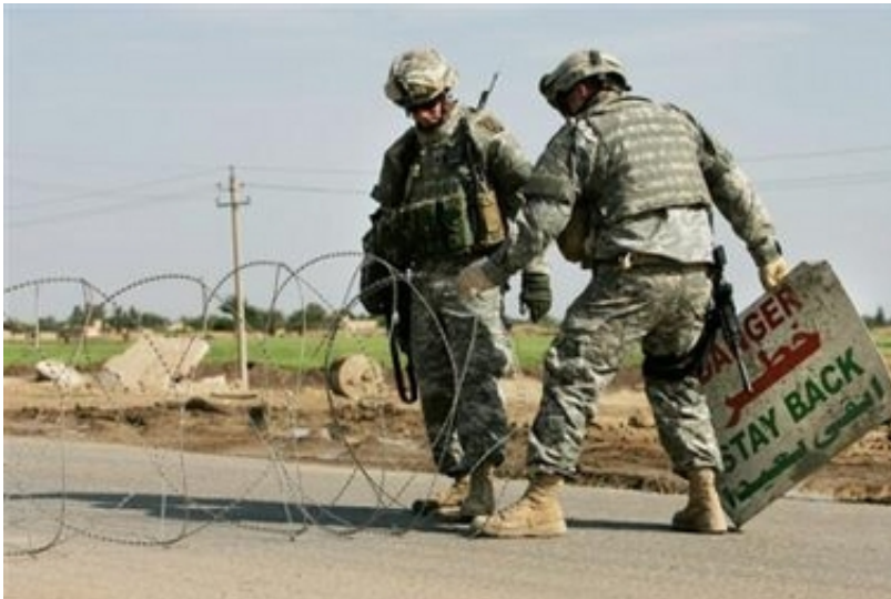
U.S. Army Sgt. Scott Rebarchak, left, of Clarion, Pennsylvania and Spc. Jeremy Broadway, of Bowdon, Georgia, construct a checkpoint near the airport in Baghdad, April 4, 2006. (AP Photo/Jacob Silberberg)
