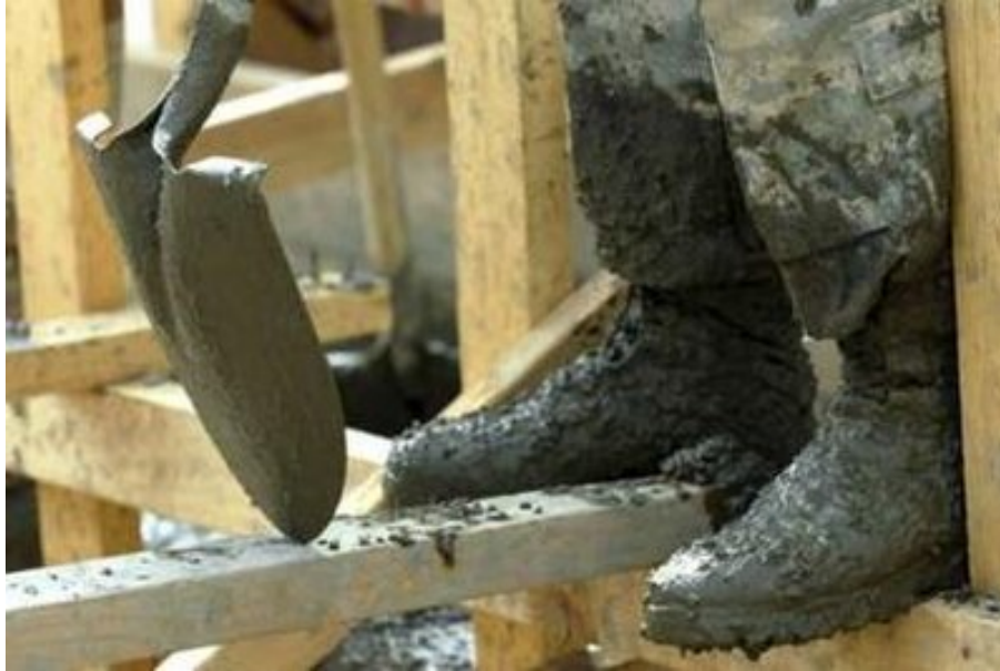
A U.S. soldier from 46th Engineer Battalion stands on a frame, above cement which was just poured in for a vehicle maintenance ramp, at Al-Muthana Airfield in Baghdad March 8, 2009. REUTERS/U.S. Army/Staff Sgt. Mark Burrell/Handout
