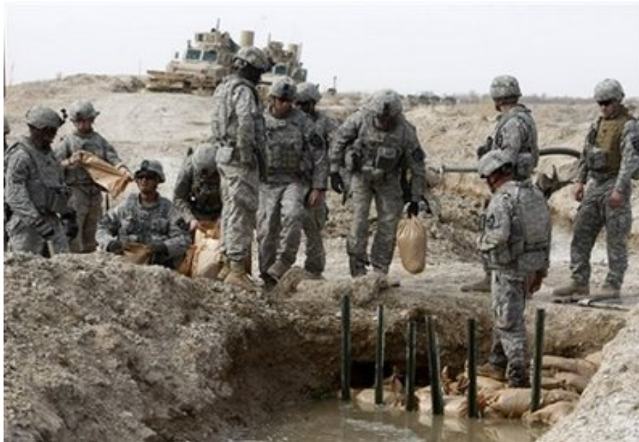
U.S. soldiers of the 562 Engineer Company, 5th Brigade, 2nd Infantry Division, work on a bridge over a canal west of Lashkar Gah in Helmand province, southern Afghanistan, Feb. 11, 2010. (AP Photo/Pier Paolo Cito)
